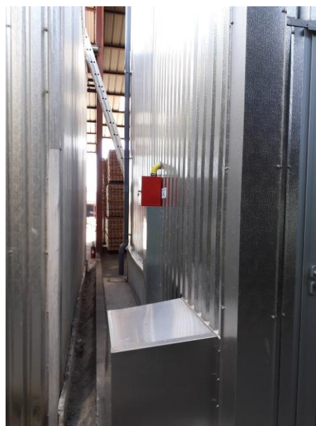
Figure 9 : Vanne alimentation gaz
